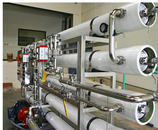
EPS biofouling on RO membrane skids raises pressure drop and cuts flux long before scale does.
