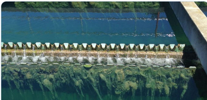
BEFORE — algae overgrown on the clarifier weirs.
